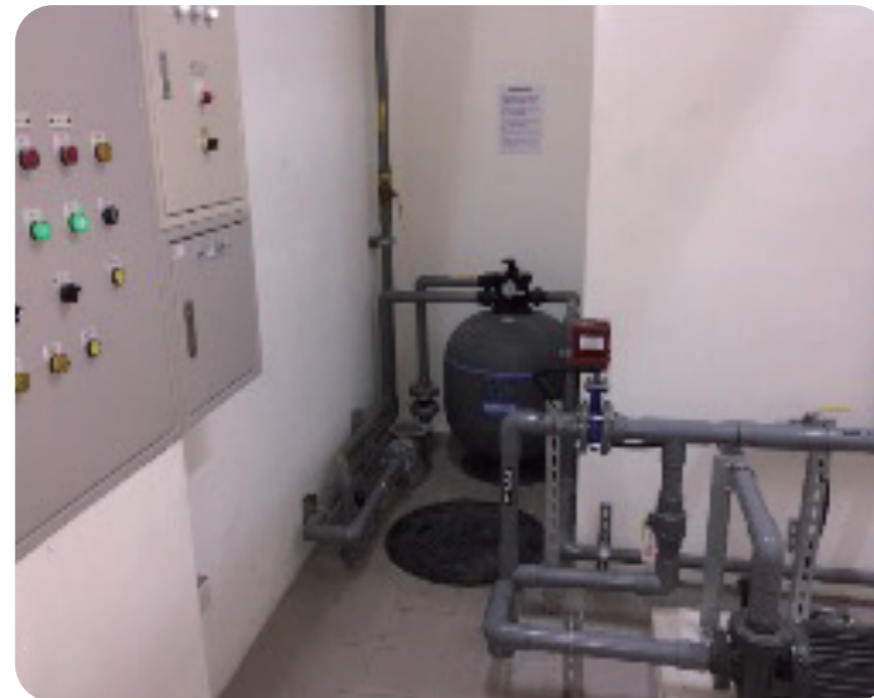
Rainwater harvesting and storage system
