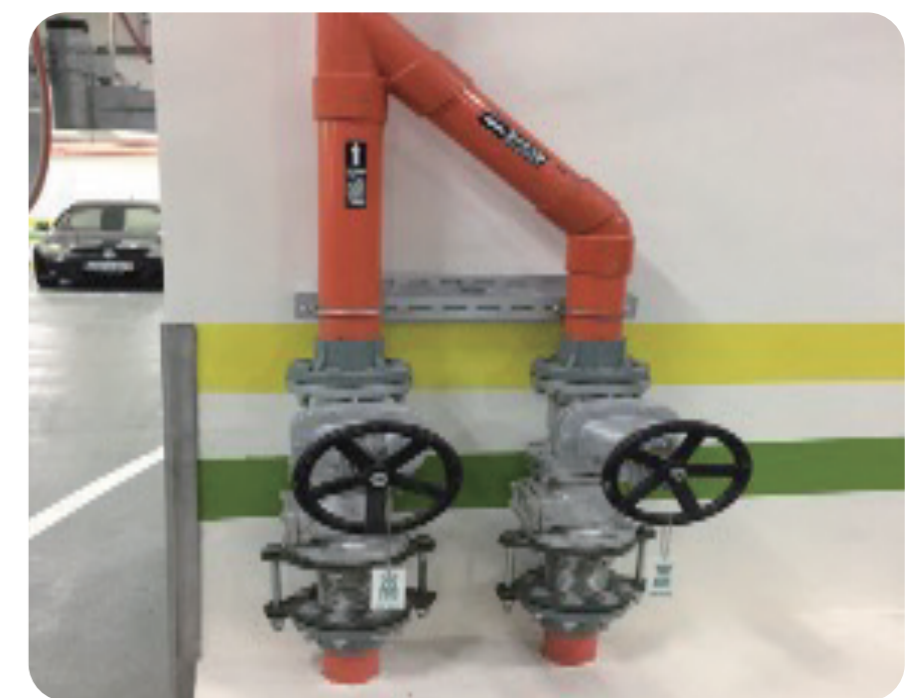
Wastewater treatment: dedicated pipelines for wastewater
