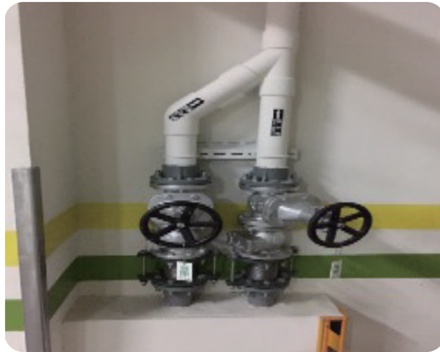
Wastewater treatment: dedicated pipelines for rainwater
